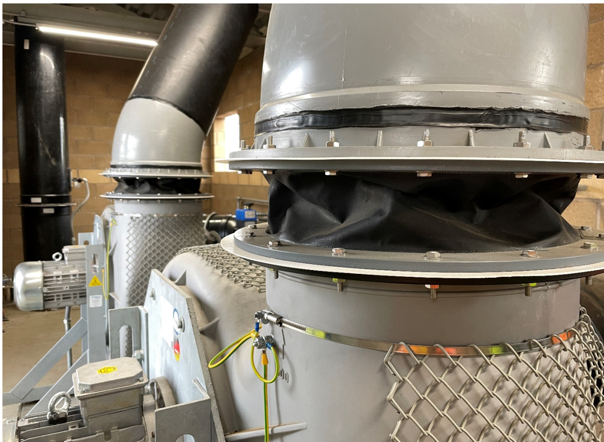
(Argo Drain Sub Basin Facility)
