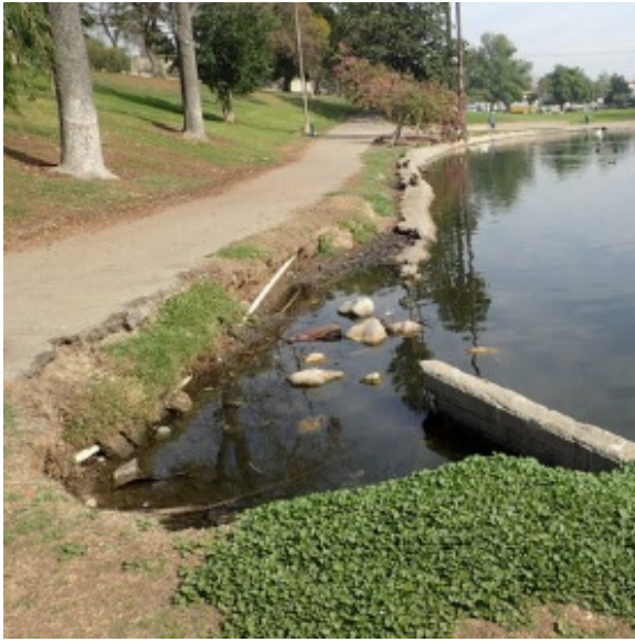
Figure 2-7-G. Lakeside Erosion Exposing Irrigation Lines Hollenbeck Park Lake Rehabilitation and Stormwater Management
