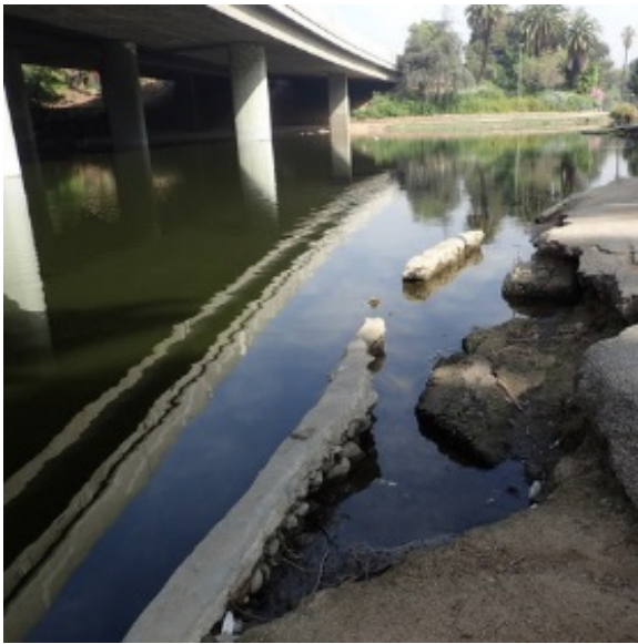
Figure 2-7-O. Lakeside Erosion Hollenbeck Park Lake Rehabilitation and Stormwater Management
