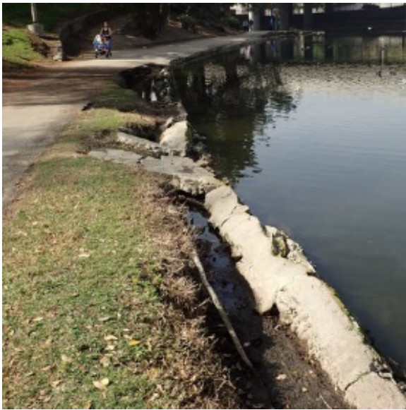
Figure 2-7-K. Lakeside Erosion Exposing Irrigation Lines Hollenbeck Park Lake Rehabilitation and Stormwater Management
