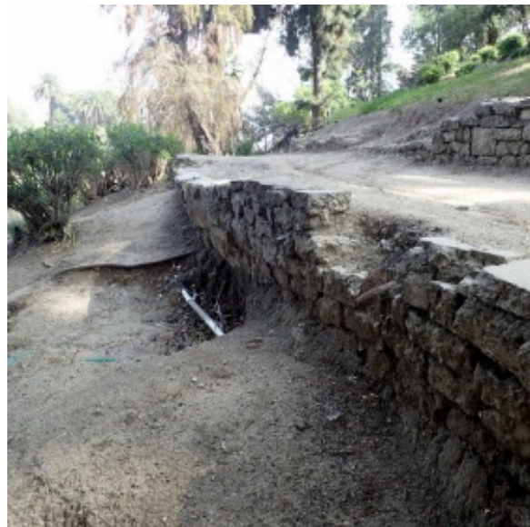
Figure 2-7-N. Hillside Erosion Exposing Irrigation Lines Hollenbeck Park Lake Rehabilitation and Stormwater Management
