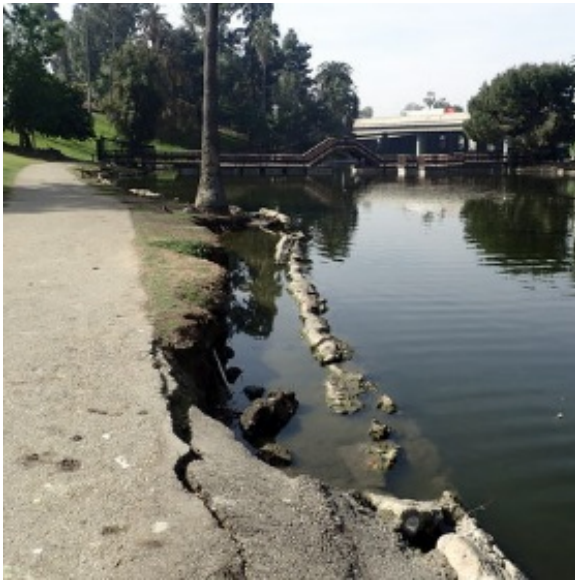
Figure 2-7-I. Lakeside Erosion Undermining Pavement and Tree Hollenbeck Park Lake Rehabilitation and Stormwater Management
