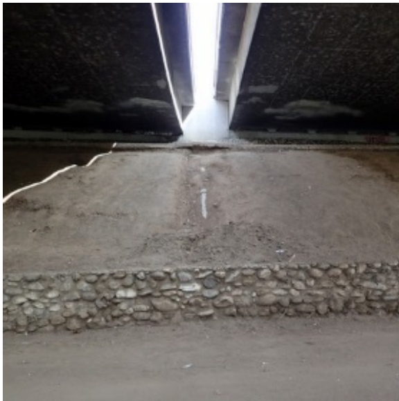
Figure 2-7-A. Erosion Between Bridge Decks Exposing Pipe Hollenbeck Park Lake Rehabilitation and Stormwater Management
