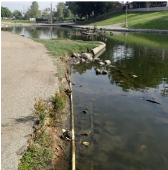
Figure 2-7-E. Lakeside Erosion Exposing Irrigation Lines Hollenbeck Park Lake Rehabilitation and Stormwater Management
