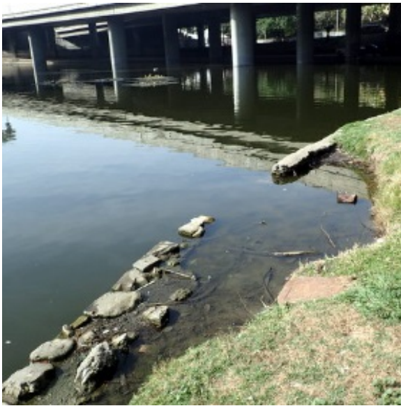
Figure 2-7-C. Lakeside Erosion Exposing Utility Vault Hollenbeck Park Lake Rehabilitation and Stormwater Management
